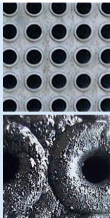
Top: Heat exchanger operating with OASE: Corrosion completely avoided Below: Not using OASE
